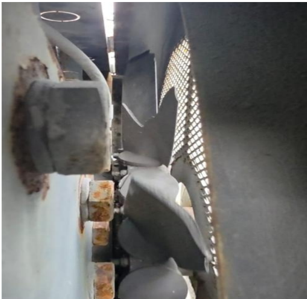
Broken Blades, Before
