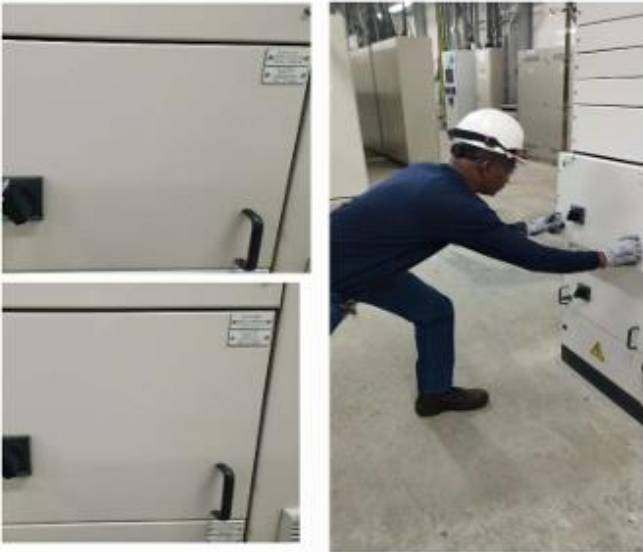
RACK IN 713CV9001- 713CV9002
